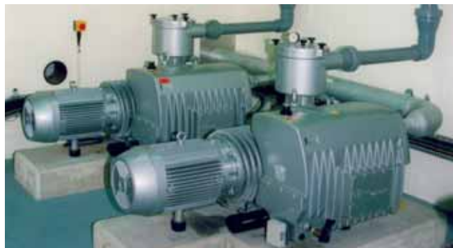
On left: pipe vacuum functioning. Above: vacuum plant.
