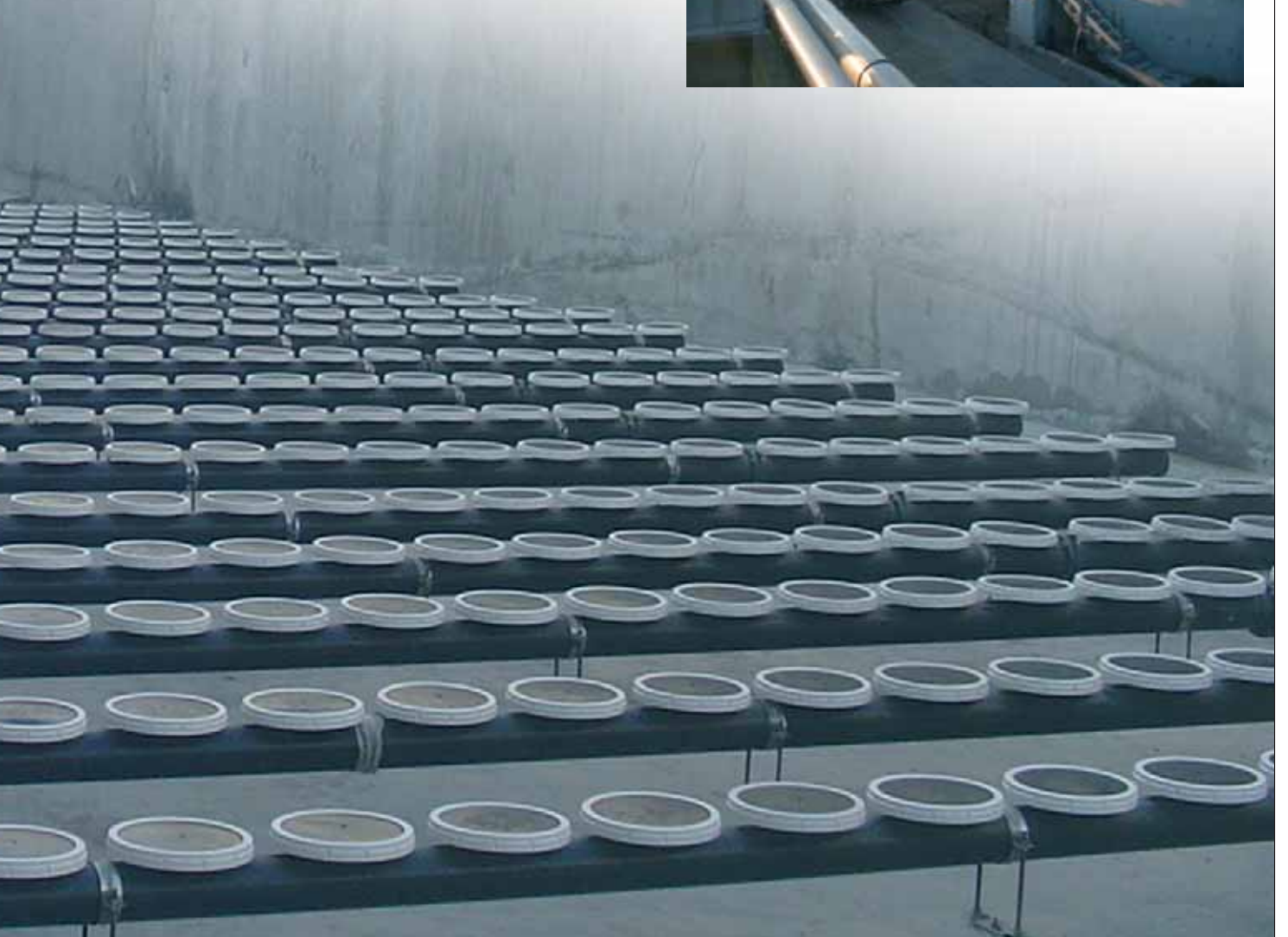
Plant servicing a textile manufacturer
