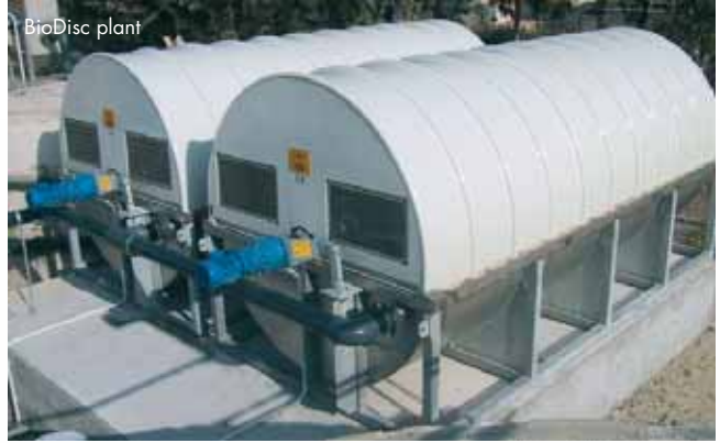
Civil works plant
