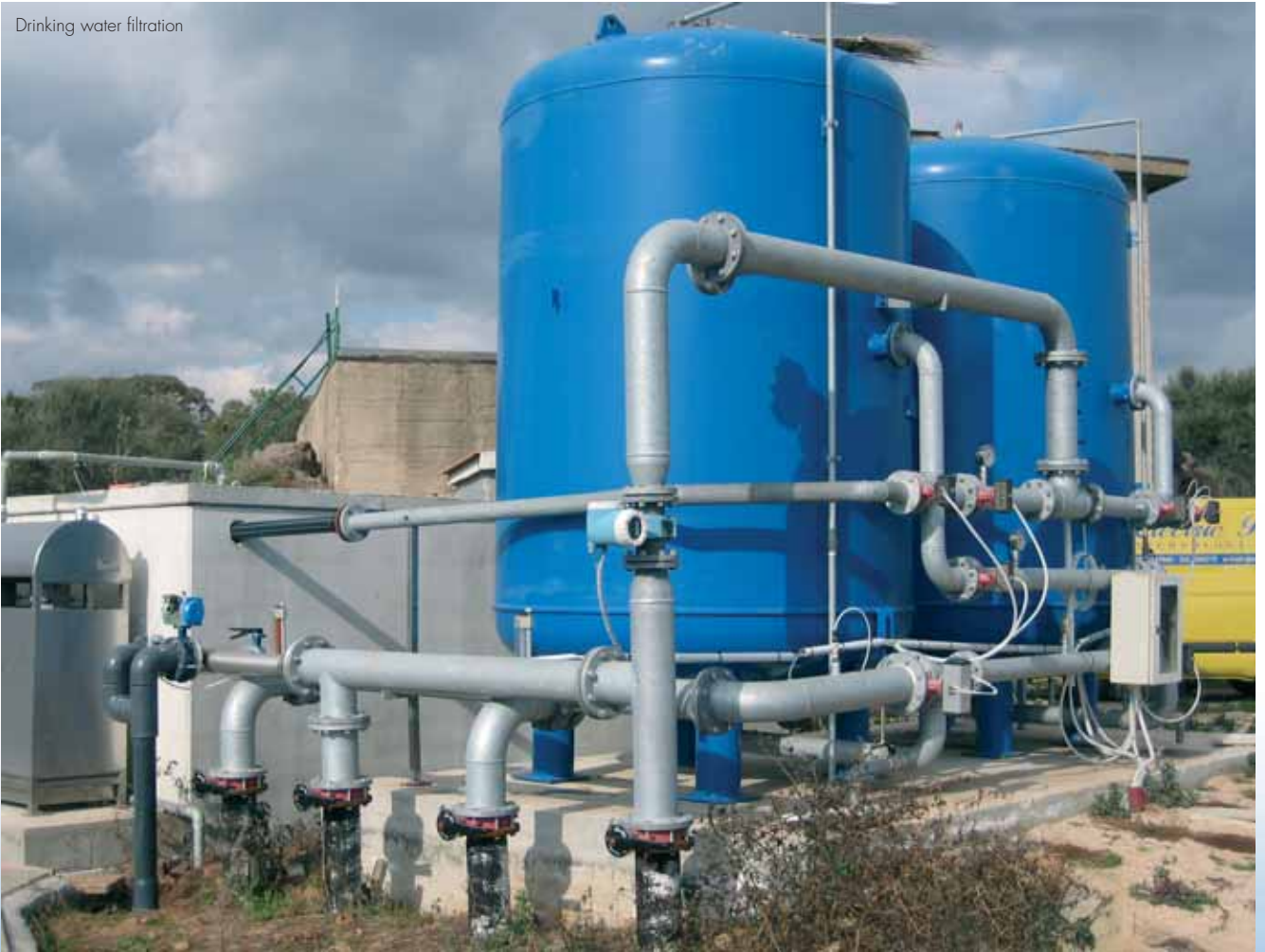
Drinking water filtration
